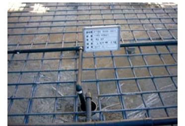
| Geo-thermal electricity system 1 |
